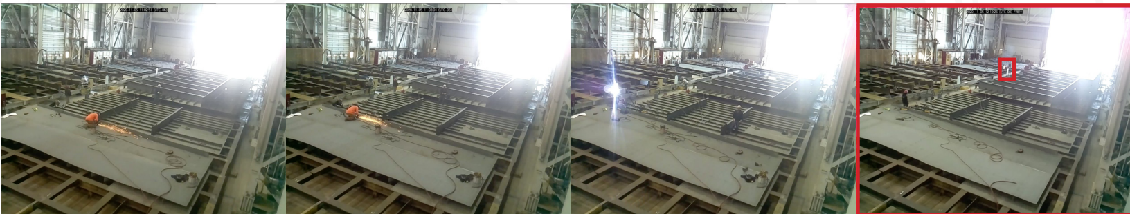
BlackStarTech's Robotic Fire Watch Series can differentiate between heat sources due to welding and mechanical cutting versus flames.
