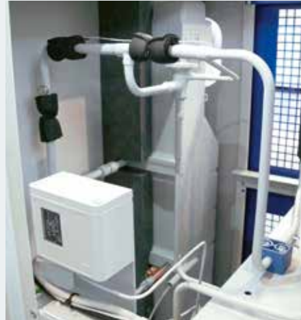
Inside of coated refrigeration dryer
